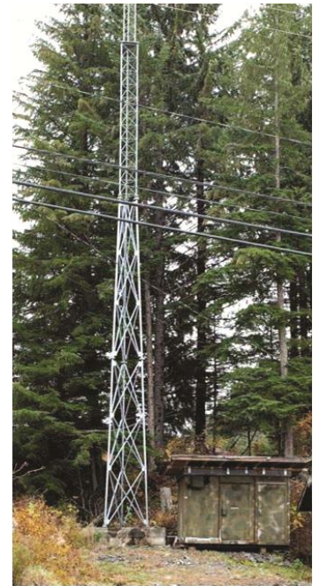
Radio Tower Serving Wrangell, AK
